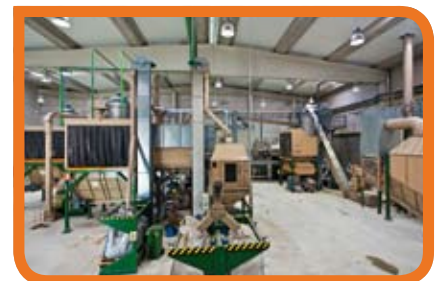
CB2G BIOMASS PRE-TREATMENT UNIT INCLUDING BIOMASS TORREFACTION PILOT PLANT
